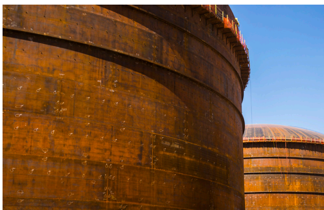
Figure 1. 50 000 t double containment ammonia tanks showing points of non-destructive examination (NDE) inspection to confirm quality construction.
